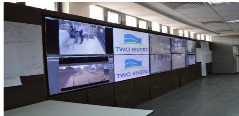
Security Operations Center
