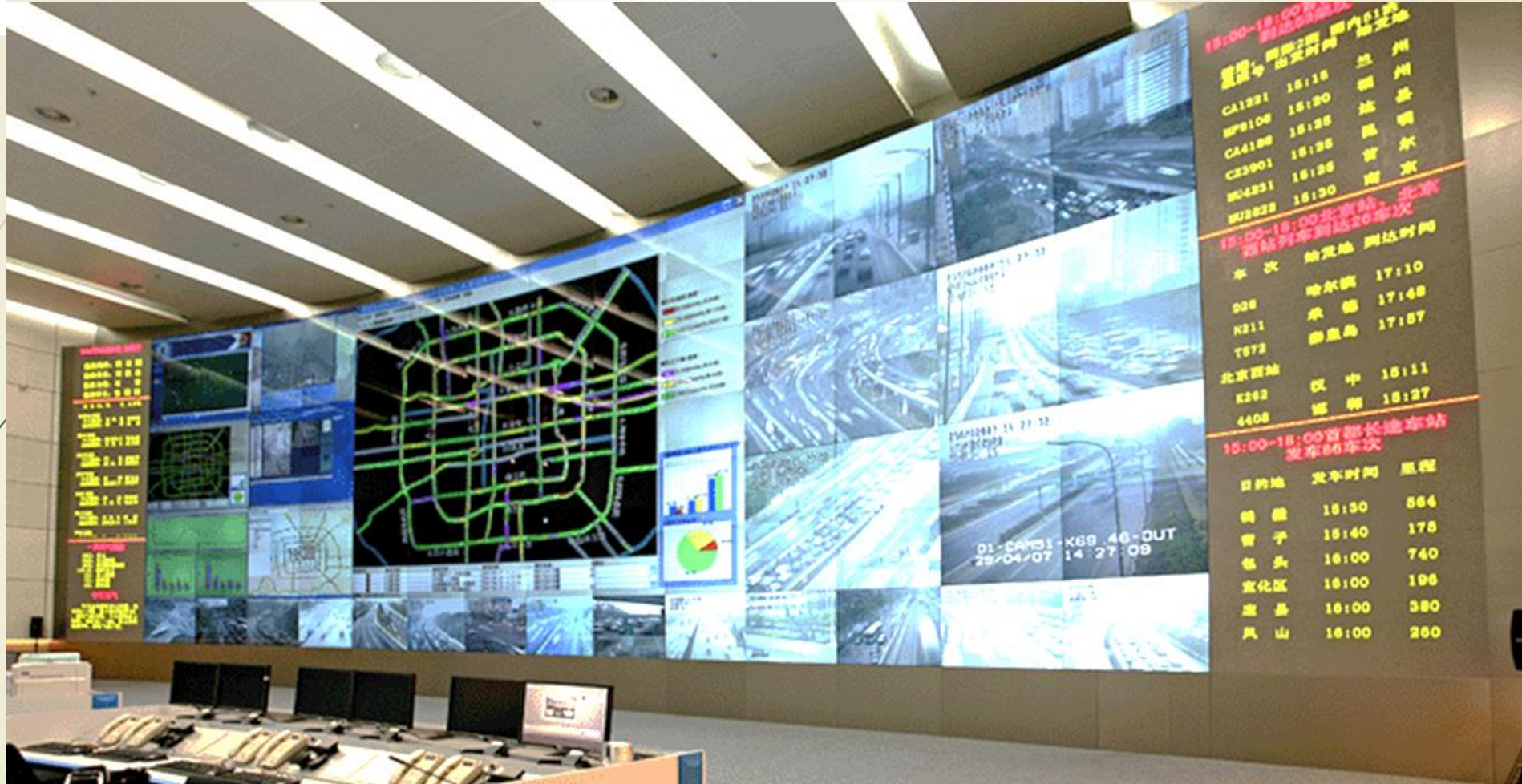
ITS... Command Control Center for Nairobi Western ring Road under installation and testing at KURA HQs
